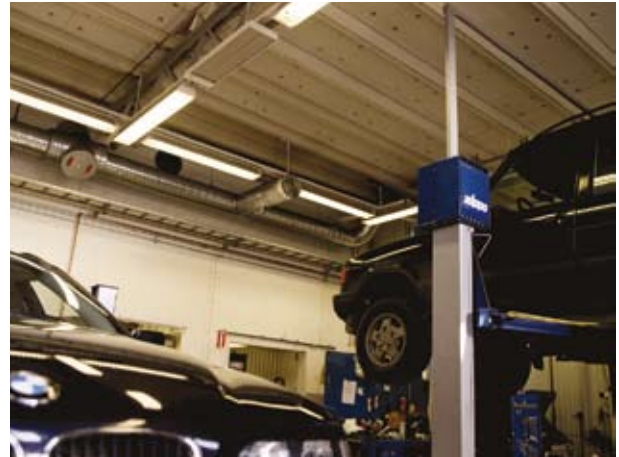
EZF blend in discreetly with the electrical fittings at BMW Group outside Stockholm.
